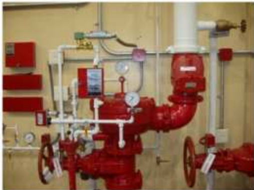
A sprinkler system pump and valves
